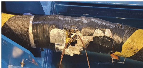
Fig. 3. Temperature sensor insertion section after dismantling the submarine cable.
