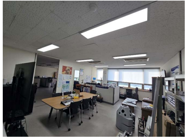
Fig. 2. Flat-panel LED lighting installed office.
