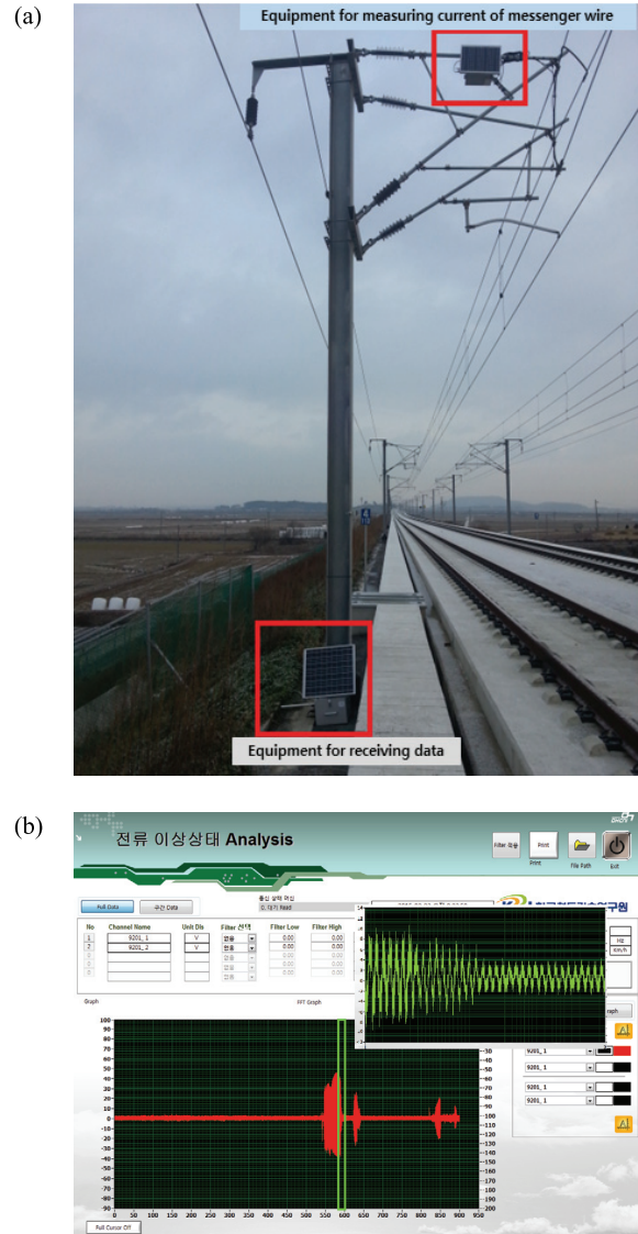
Fig. 1. Picture of current monitoring system, (a) installation of current monitoring system on OCL (overhead contact line) in Honam high-speed line and (b) program for analysis of current.
