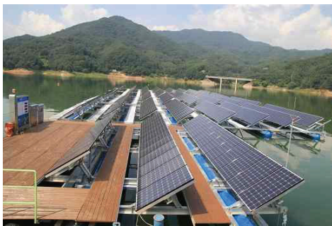
Fig. 1. Floating photovoltaic (PV) system of 100 kW installed at Hapcheon dam in 2011.
