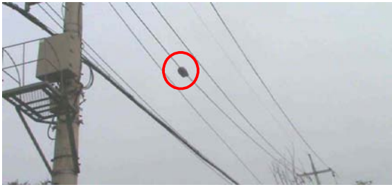
Fig. 7. Field test for overhead distribution power lines.
